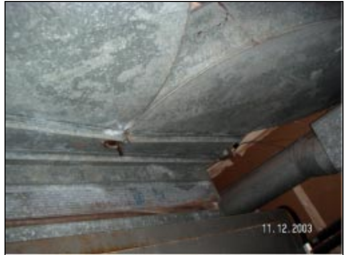
Fellowship Dual Air Supply—Poor Condition.
